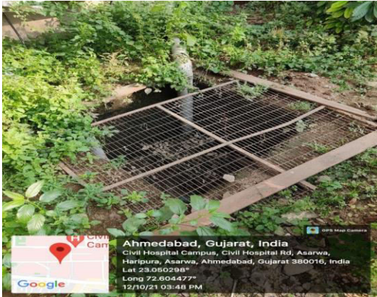
Rain water harvesting system
